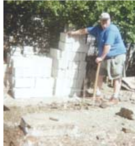
Jay Decker piles cinder blocks in preparation for laying the home's foundation.
