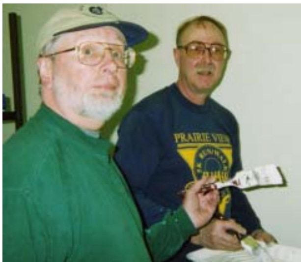
Joe Greene (left) and Fr. Stan Uroda, SVD, apply the first coat of paint to a room inside the church hall.
